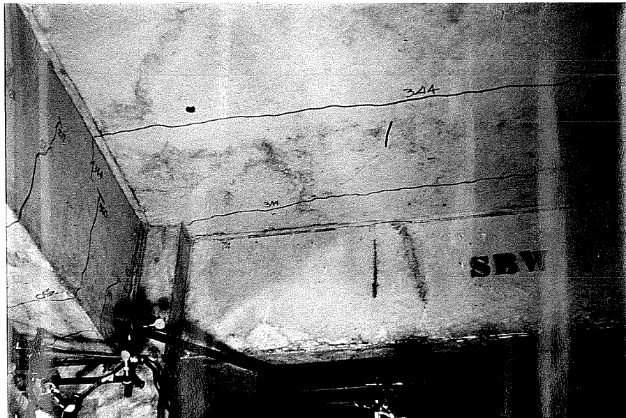
Fig. 4.10 Flexural cracking in the slab
