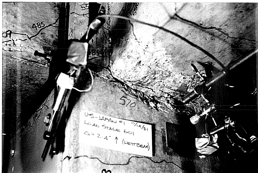
Fig. 4.20 Deterioration in hinging zones, west beam
