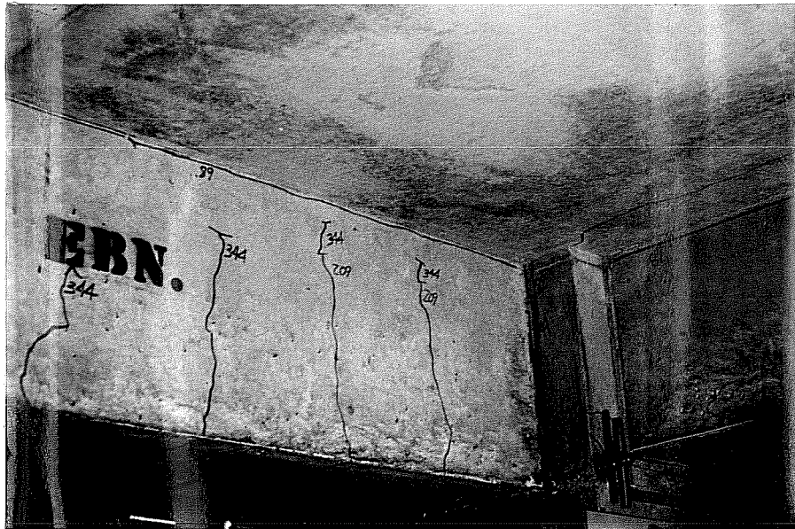
Fig. 4.9 Flexural cracking in east beam
