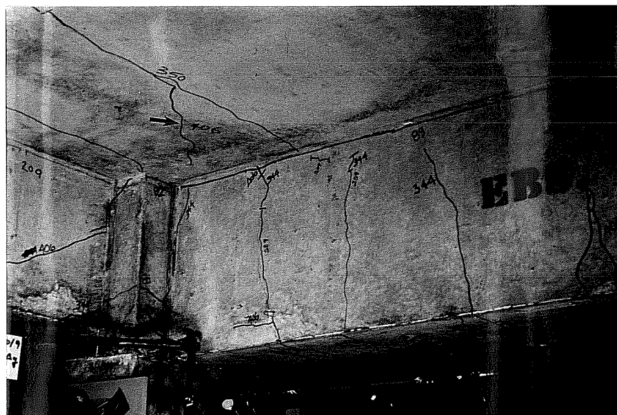
Fig. 4.12 Crack propagating diagonally in slab
