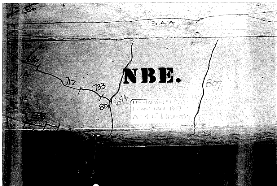
Fig. 4.26 Vertical cracks in north beam
