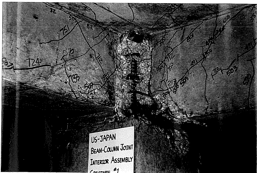
Fig. 4.28 Deterioration of NW joint region
