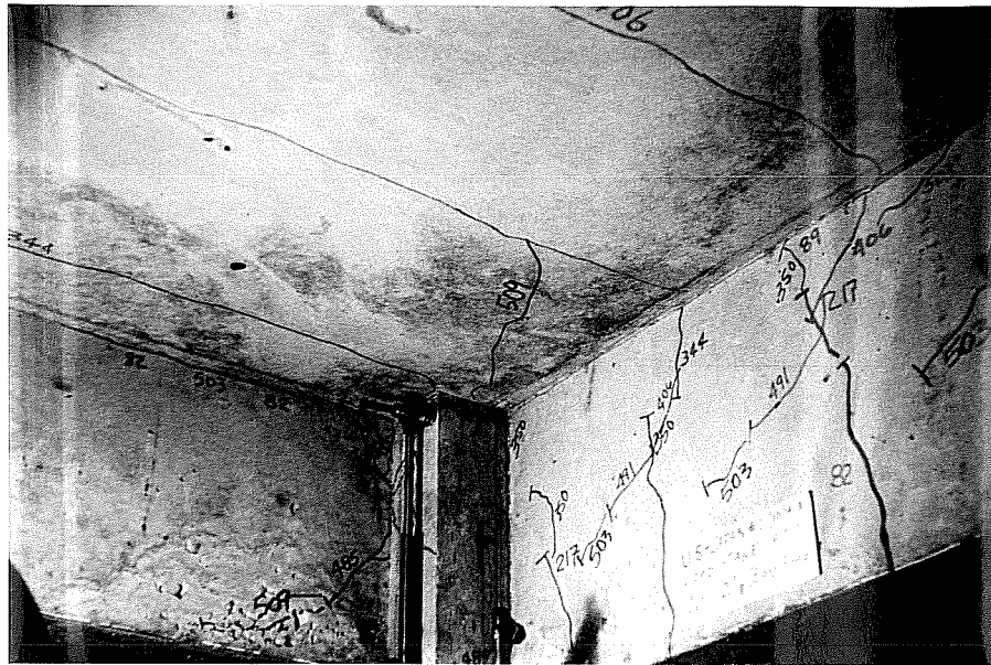
Fig. 4.19 Crack patterns at load stage 509
